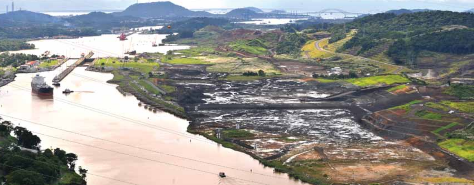
View of the work under the third phase of the dry-excitation from the Centennial Bridge.
