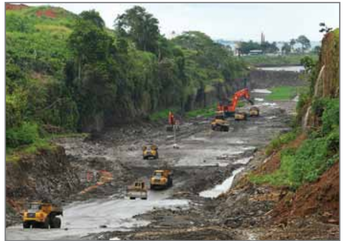
Dry-excavation work in the area of the Third Set of Locks chambers on the Atlantic side.
